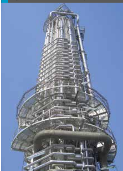
Fig. 24: Nitric acid absorption tower
